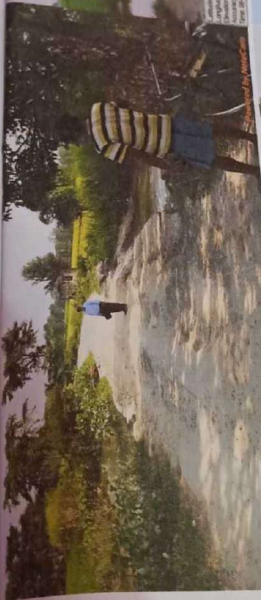
Time: 02-10-2020 14:24 Note: pwd road to dhamaura flood damage in near bhatani 1
